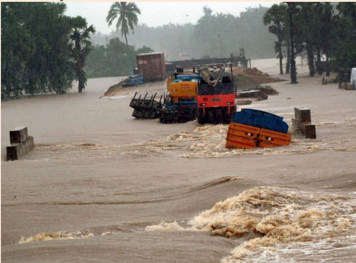
A washed-away road in Suchindram at flood-hit Kanyakumari. (PTI Photo) – Source: rediff.com, news dated 1 st Dec 2017
