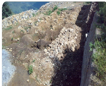
Uttarakhand: PHC Manthat, Dehradun under construction since 2005 (Rs. 56.10 lakh released till March 2008)
