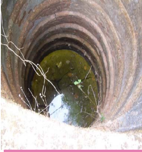
Unhygienic water storage facility at Sub Centre Madavoor, Kerala
