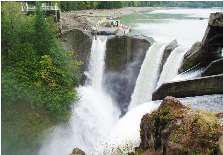
Figure 9. Glines Canyon Dam on the Elwha River during the dam removal process. Photo credit: USGS, Source: https://www.usgs.gov/center-news/new-report-synthesizes-us-dam-removal-studies
