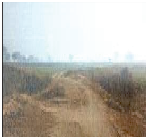
Photograph No. 3.13.2: Approach road not constructed (photographed in December 2018)
