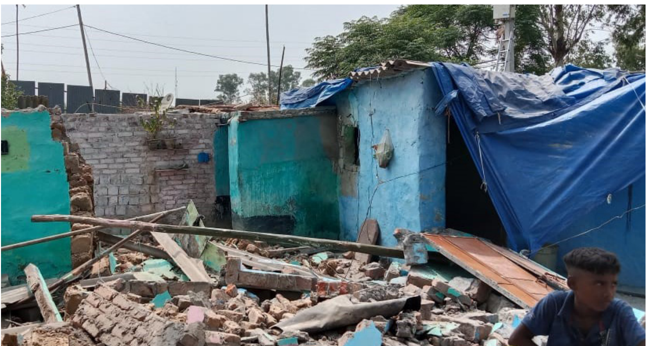
Demolished homes in Gyaspur, Delhi
