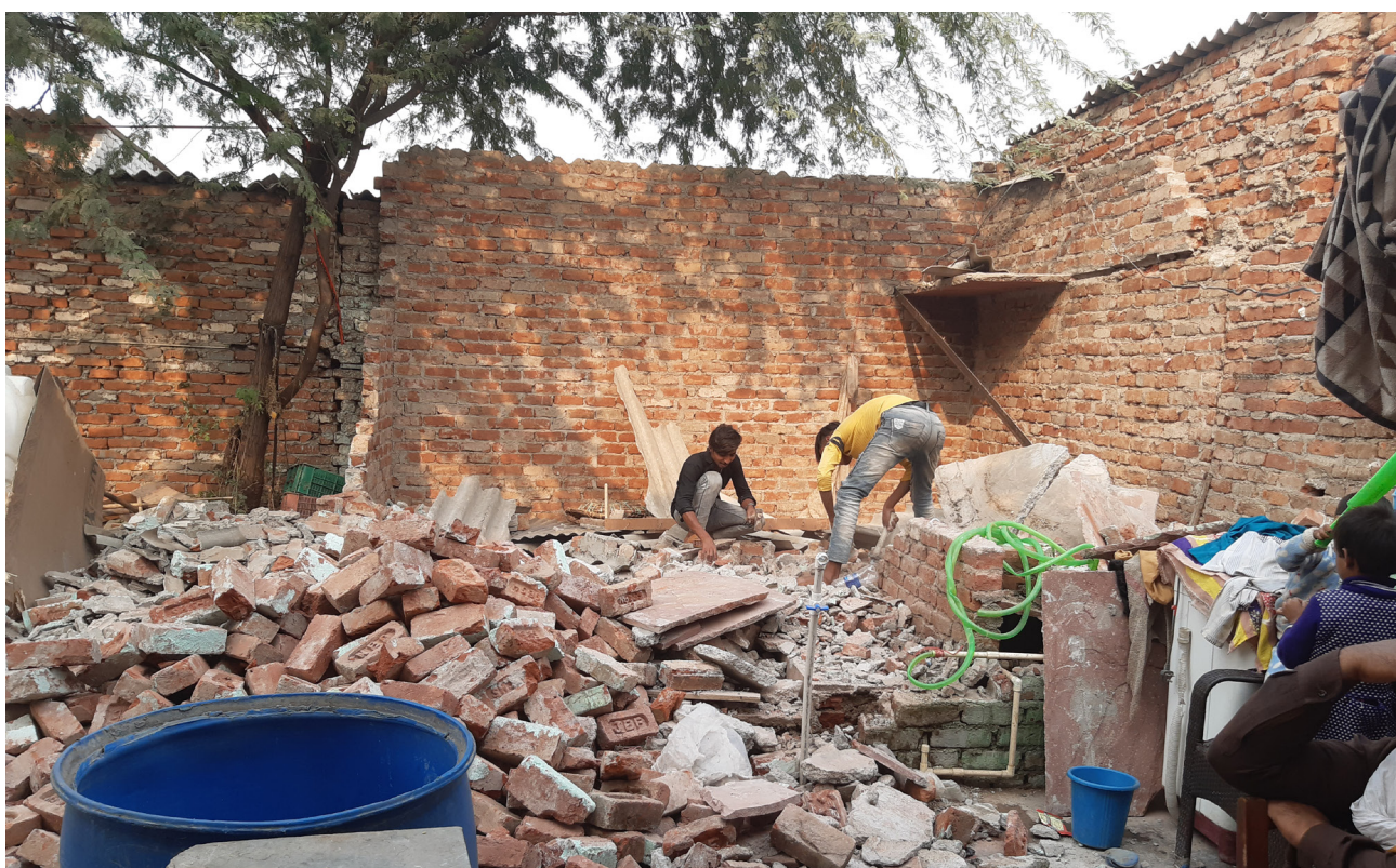
Affected persons collecting their belongings after the demolition of their homes in Rangpuri Pahadi, Delhi
